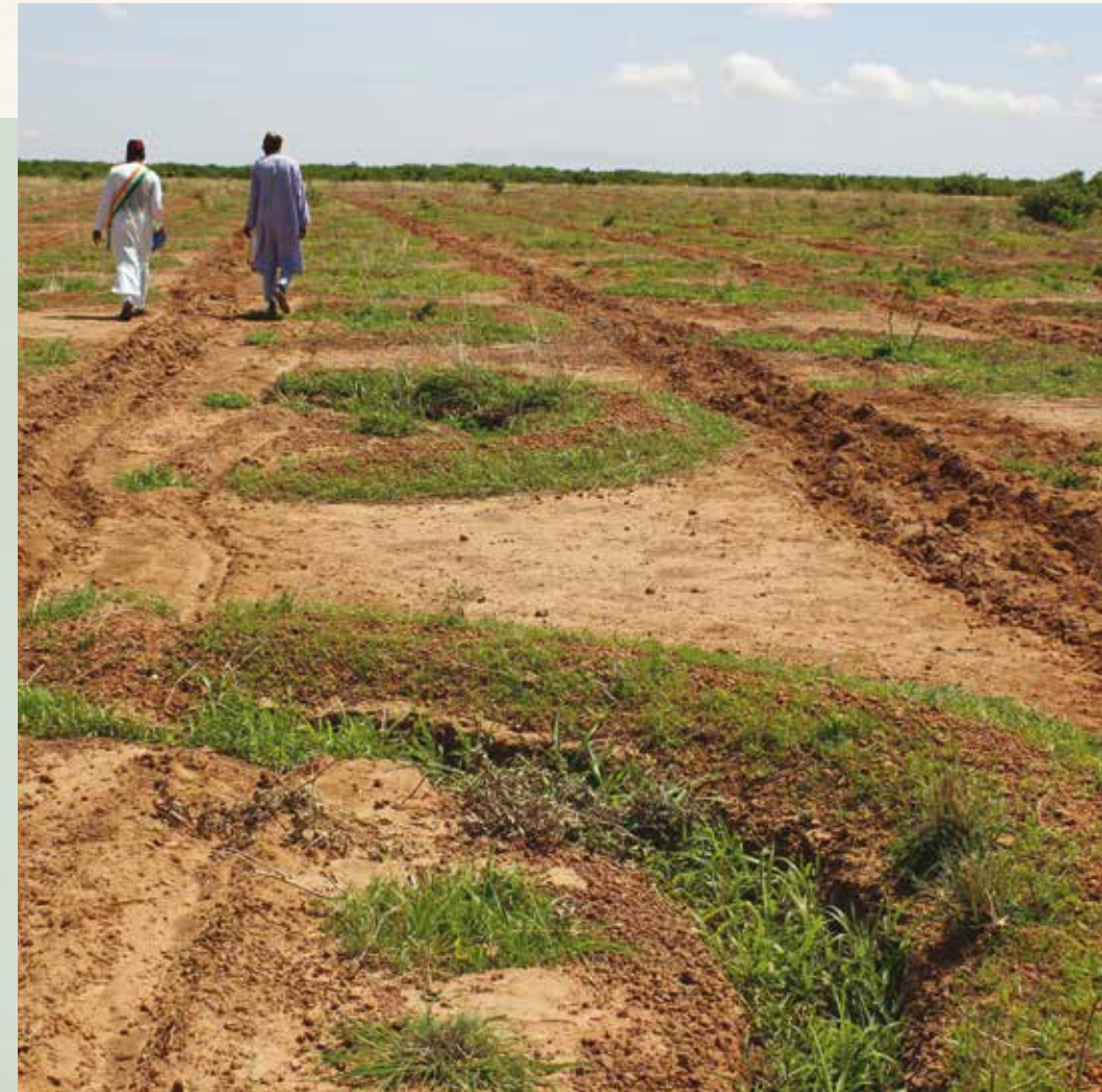
Half-moon structures to combat desertification, recover desert land and preserve crops, Niger
