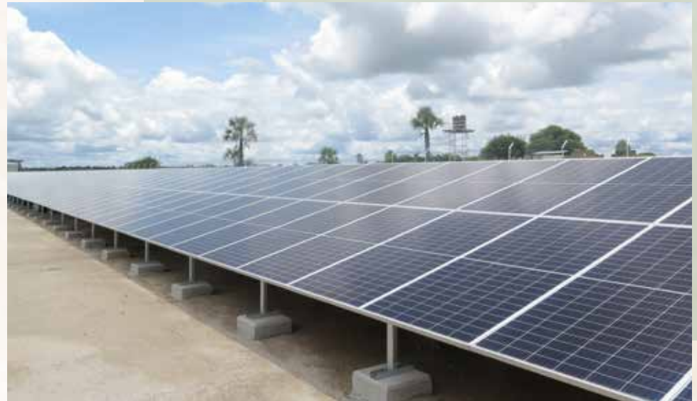
Solar panels for pumping water, agricultural farm, Namibia
